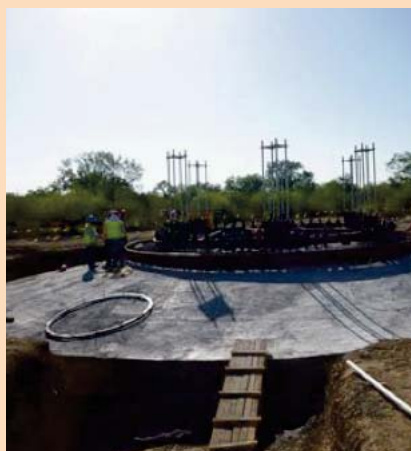
Ventika Wind Farm
